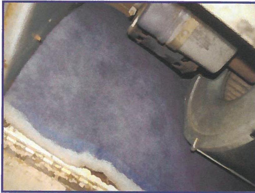
LIBRARY SEMINAR ROOM-UNIT COIL/DRAIN PAN
