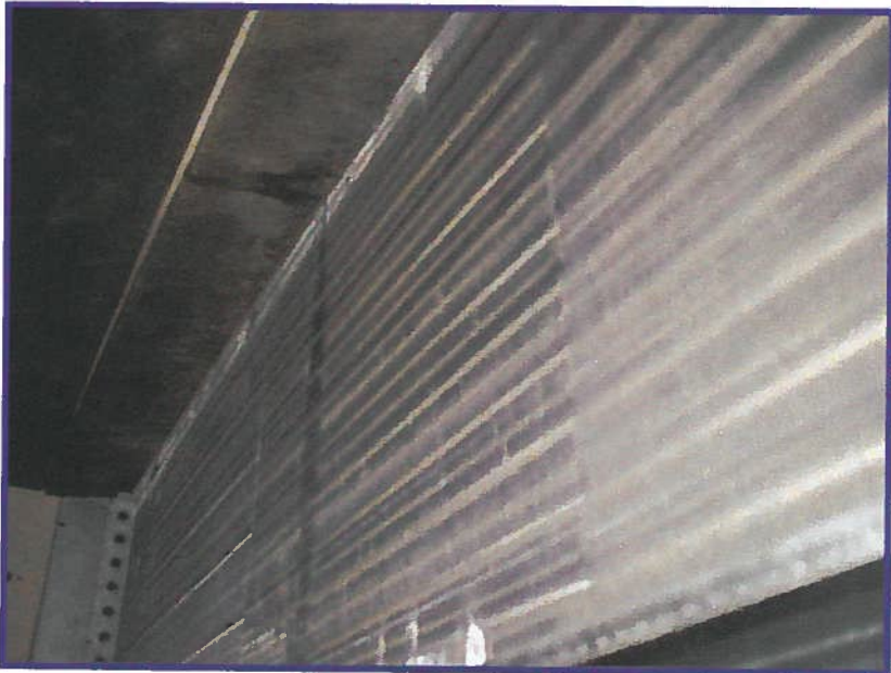
TEAM ROOM-UNIT COILS DOWNSTREAM
