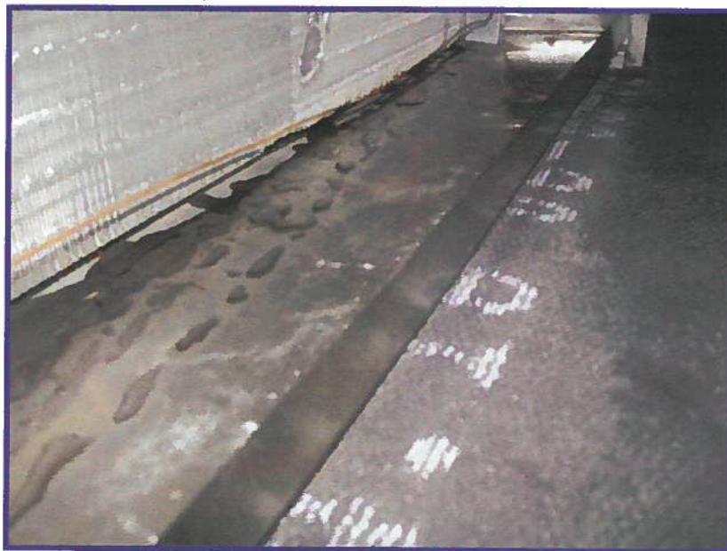
ROOM # 137-UNIT BLOWER
