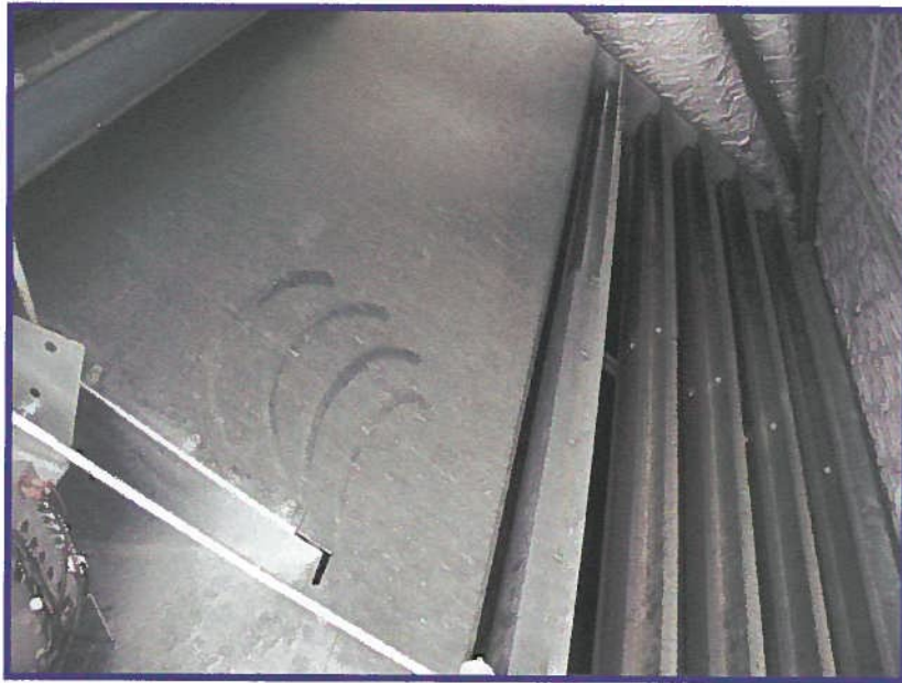
RTU -GYMNASIUM FARTHEST FROM FLAGPOLE -FILTERS
