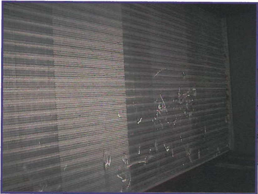
AHU # ?-CAFETERIA -BLOWER
