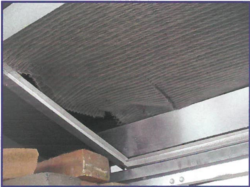
RTU -GYMNASIUM CLOSEST TO FLAGPOLE –OUTSIDE AIR DAMPERS-NO UNIT #
